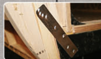
HURRICANE STRAP REINFORCED ROOF & WALLS
